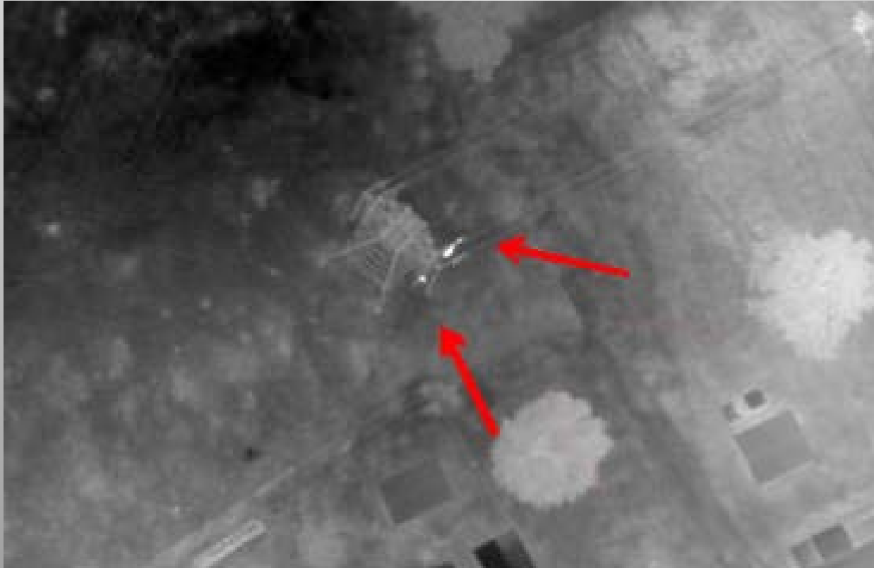
Hot spots on a high voltage transmission line
